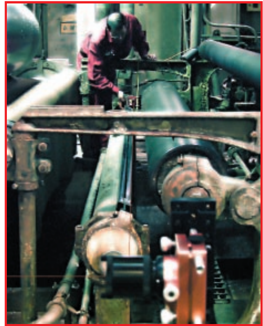
Roll parallel measurements being done by plant maintenance personnel during an unscheduled outage.
